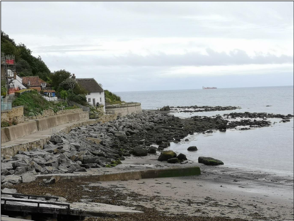
Figure 2.1. Location of new granite rock armour at the foot of the seawall, note the (colonised) natural boulders which have been placed in front of the granite rock (July 2020).
